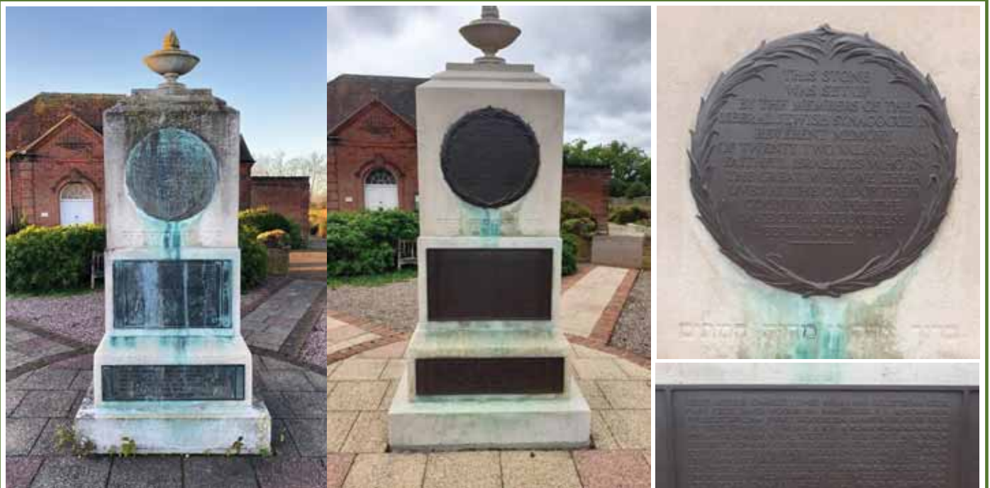
Above left: Before works (WM12103) © A Elfes Ltd, 2022 with remaining images after works © Liberal Jewish Synagogue, 2022
