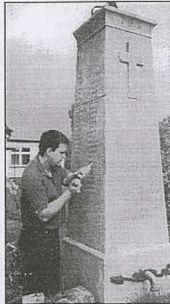
Newton War Memorial: Mark Metcalfe of contractors Rattee & Kett recuts the names - Photo by Jane Gaskell
