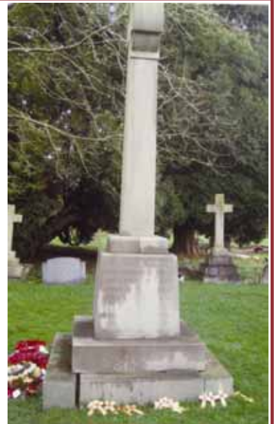
The memorial before work was undertaken with visible gaps in the joints © Caddington P. C.
