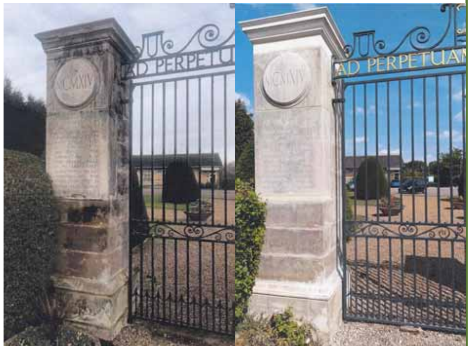
Above: Kirby Muxloe gates after works and below: pier before and after works (WM11506) © Kirby Muxloe Parish Council, 2021 and 2022
