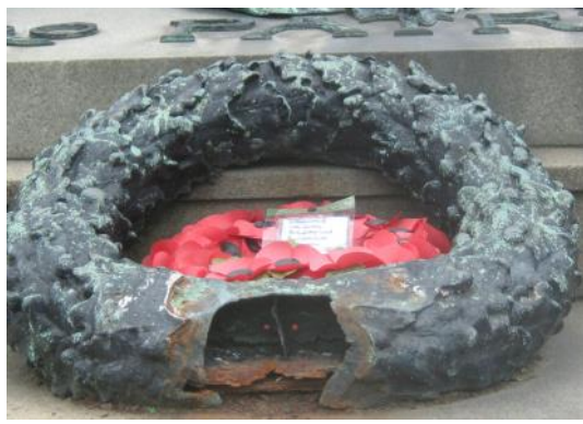
Untreated damage can speed up deterioration due to water ingress © War Memorials Trust, 2010
